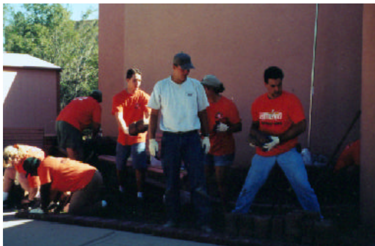
Employees from Home Depot # 3504 on Coors assist with a new patio for Casa Esperanza. Materials were donated by Pavestone Co. of Colorado, and project director Ben Hilliard (white shirt) trained the willing workers to set the pavestones. The result is a terrific new patio with accompanying planters, providing our families with a tranquil area - the perfect place to view the setting sun.
