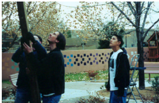
Nick Williams is assisted by friends as he began construction for a cover over the fountain courtyard. Nick created, planned, organized, sought donations for and directed the project which will serve to fulfill his requirements for his Eagle Scout status. The new cover will allow our families to enjoy this lovely area even on the hottest days.
